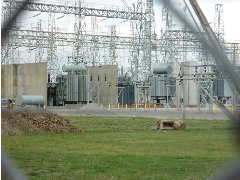
220 kV → 66 kV transformator
